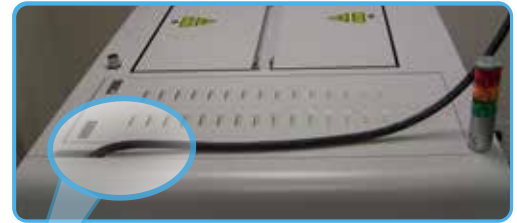
Power Supply Drop
